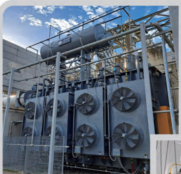
Italy ENEL Montalto di Castro Power Plant 400kV 180MVA Step-up Transformer
