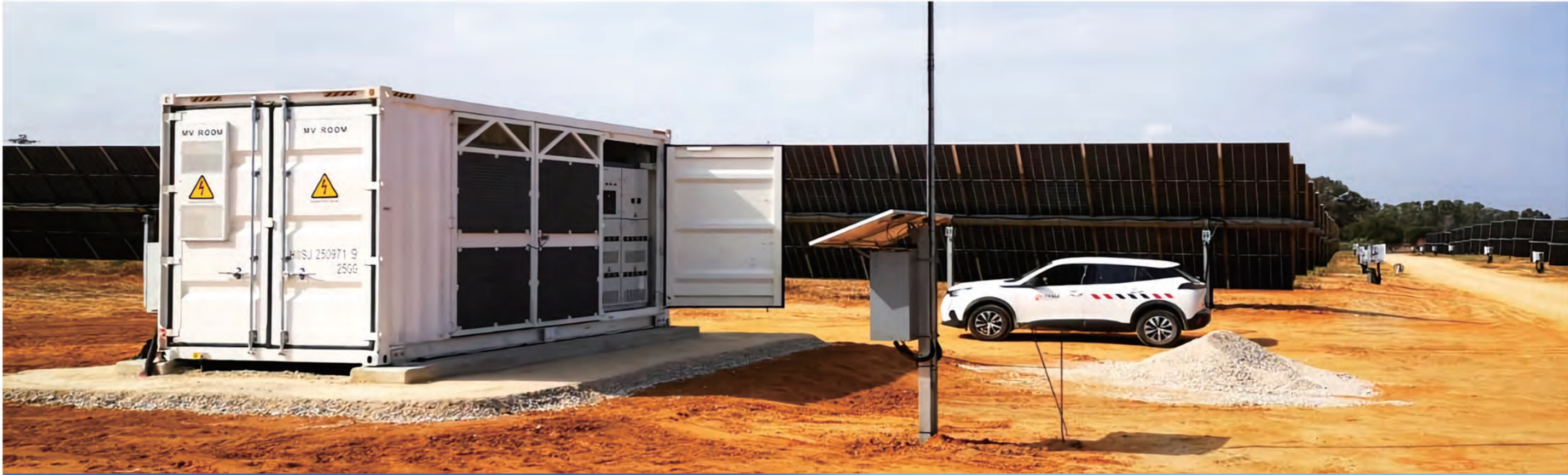
250MW High-altitude 6500kVA Container Substation in Chile
