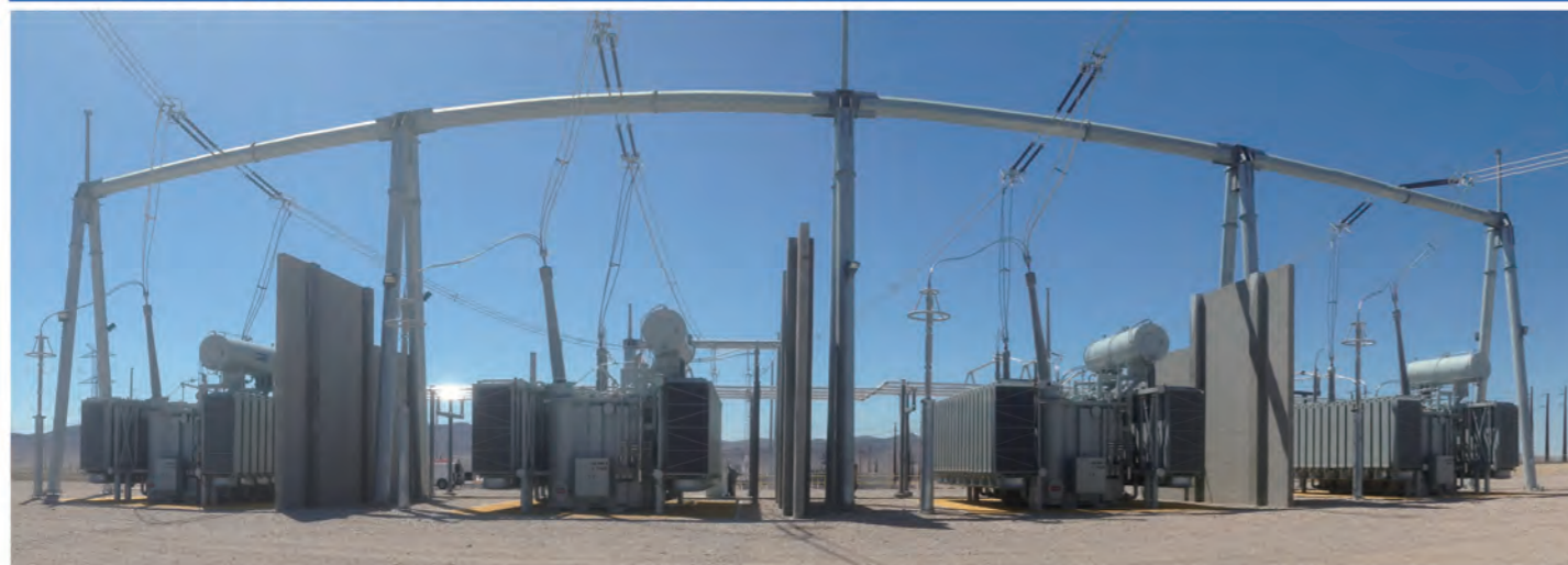
Las Vegas, USA 500MVA 525kV Single Phase Power Transformer
